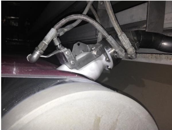
Teflon cleaning head for Dryer Fabric cleaning with HP water
